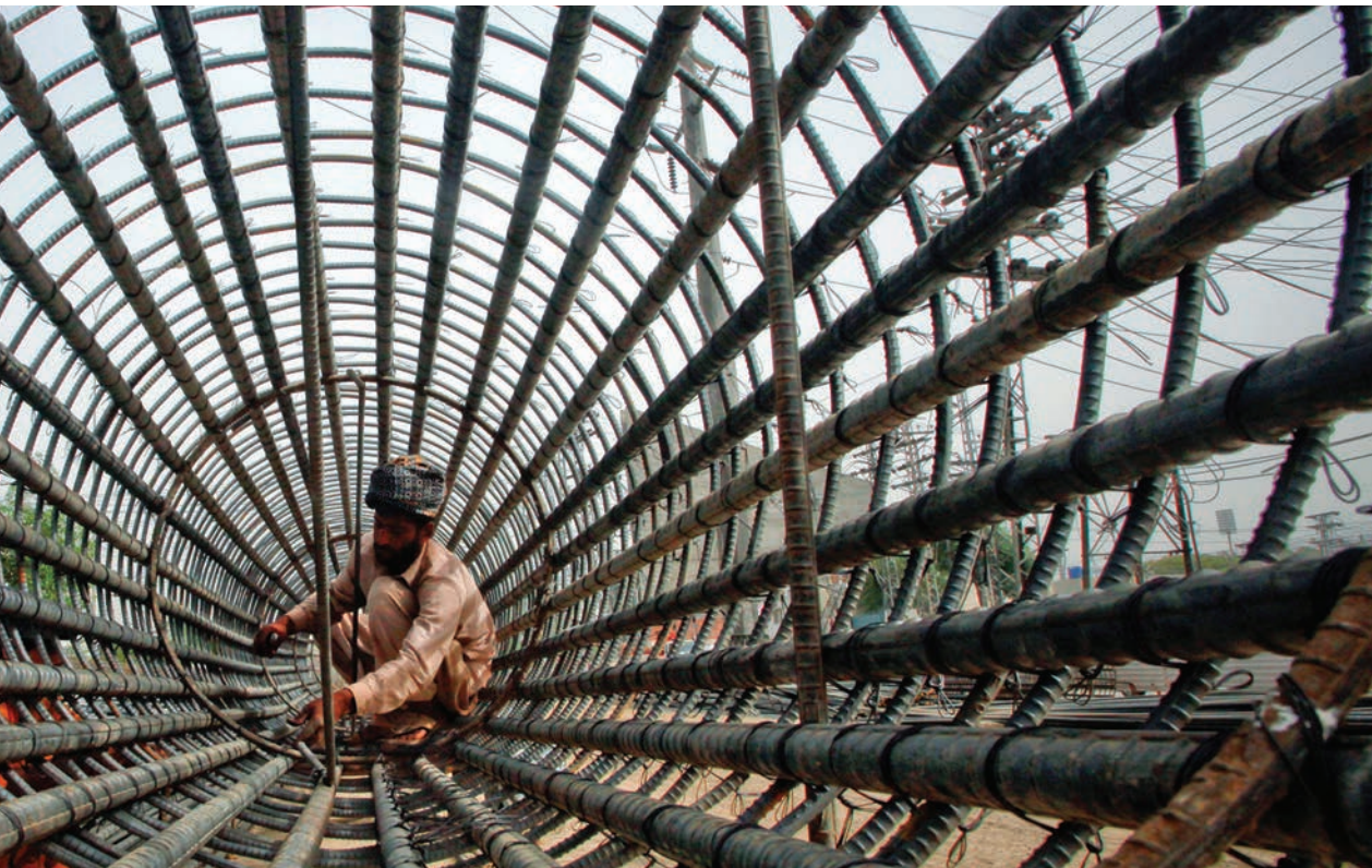
< A labourer attaches iron rods to a column at the construction site of a flyover in Lahore. REUTERS/ Mohsin Raza
